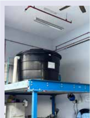
Rainwater Harvest Collection System
